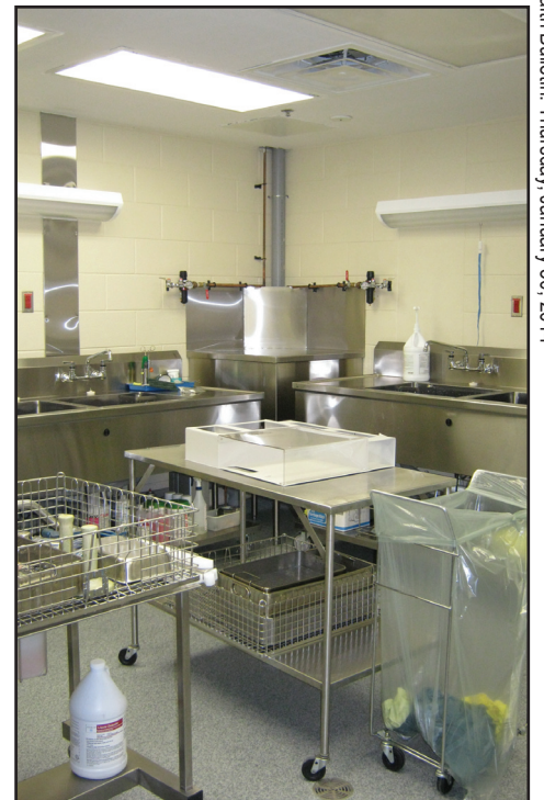
AFTER THE RENOVATION. The Medical Device Reprocessing Department at the South Muskoka Memorial Hospital Site in Bracebridge underwent a significant renovation in the summer of 2013.
